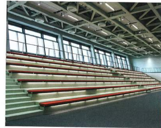
The air-conditioning outlets in the multimedia hall can be adjusted to diffuse cool air or provide direct jets of warm air.
